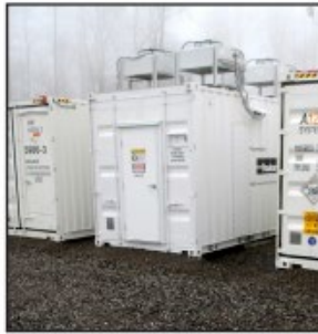
4 Megawatt PCS container (Part of 32 MW installation)
