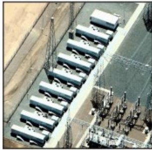
Aerial view of 12 MW installation
