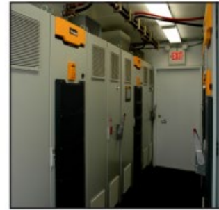
PCS interior view showing inverter stacks and connection cabinets
