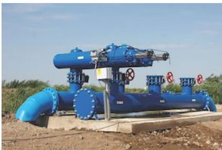
Water & Wastewater Products
