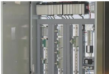
Control Panels & Systems
